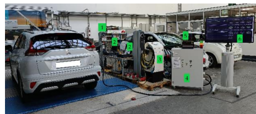
Bidirectional EV charger laboratory setup
